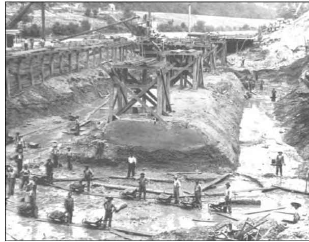
Workers excavating the abutment of Dam No. 7, loading stone on skips for hoisting and removal from the pit.
