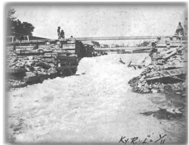
Kentucky River dams often developed leaks and required constant maintenance.
