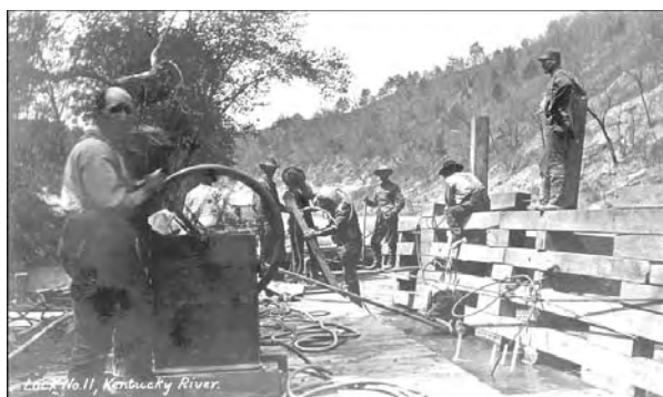
At Dam No. 11 in April 1906, a diver attaches lines to the last crib to be floated into position in the cofferdam around the dam site.
