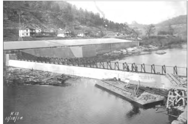
Metal trestles for the movable crest of Dam No. 13 are in place in Nov. 1914. A drift is at the left and a needle flat for maneuvering the trestles is at the right. Note the three lockhouses in the background.
